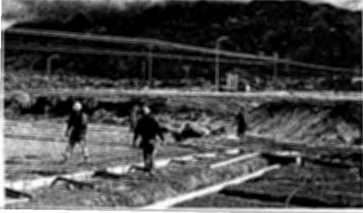
Work in Progress on the Futures for Children Learning Center on Tramway Boulevard. Scheduled to open in mid-July.
