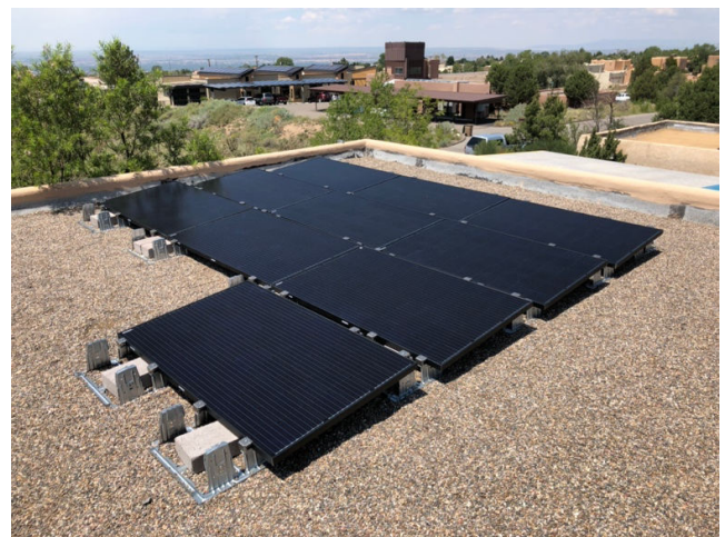
Flat-roof, ballasted PV installation not visible from the street or by any neighbors.
